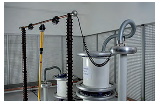
High voltage laboratory
